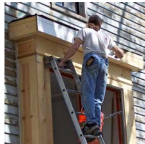
Rehabilitation of a house that was once-threatened by demolition in Fort Wayne's West Central Historic District.
