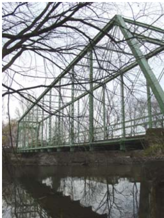
Van Zile Road Bridge(1883) crosses the St. Joseph River, north of Leo-Cedarville. A Whipple through truss iron bridge by the Massillon Bridge Co.; it is the only example in Indiana.
